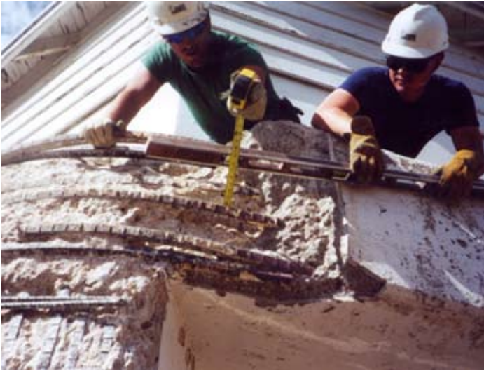
Before: Structural damage to concrete water reservoir. --- Mesa Verde National Park
