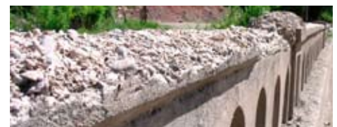
Before: Damage CDOT Hwy 145
