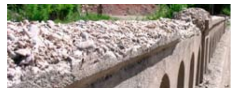
Before: Damage CDOT Hwy 145
