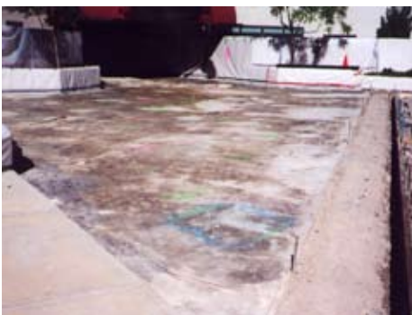
Before: Repair of concrete deck over Parking garage at Horizon Towers. --- Grand Jct. CO.
