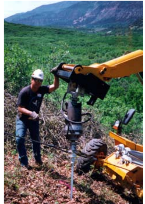
Helical piers for new 12" water line located on a mountain slope, approximately 1,400 ft. above valley floor. --- Paonia, CO.
