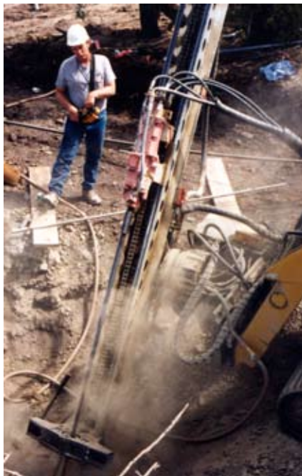
Installing rock anchors on mountain peak for television tower foundation. --- Grand Junction, CO
