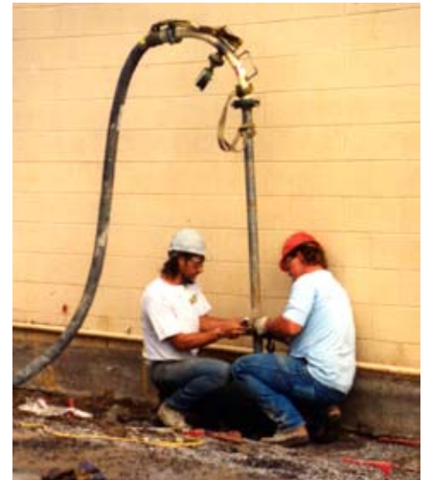
Compaction grouting used to raise and stabilize a retail center. -- Grand Junction, CO
