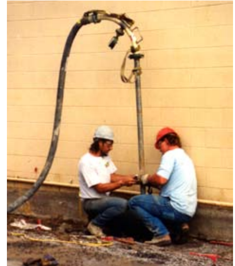
Compaction grouting used to raise and stabilize a retail center. -- Grand Junction, CO
