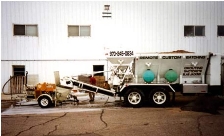
On site batching of zero slump grout using a high-pressure pump equipment.
