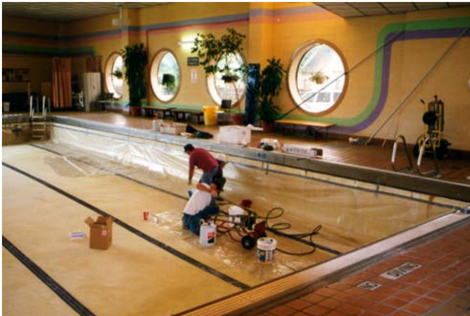
Sealing cracks in pool at Hilltop Rehabilitation Center Pool. ---Grand Junction, CO
