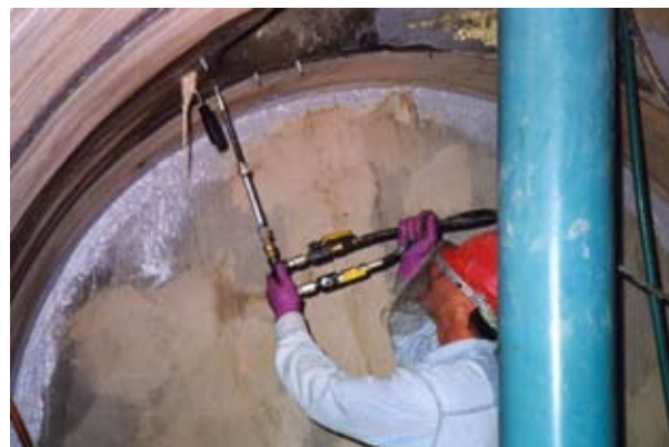
Polyurethane grout injection to seal ground water from Cliton Water District underground utility vault. ---Clifton, CO
